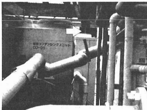
Figure 3. Failure at pipe support
