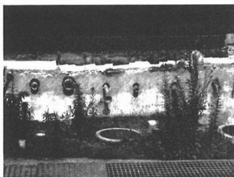
Figure 6. Pipes fractured at the connection point of the building and soil
