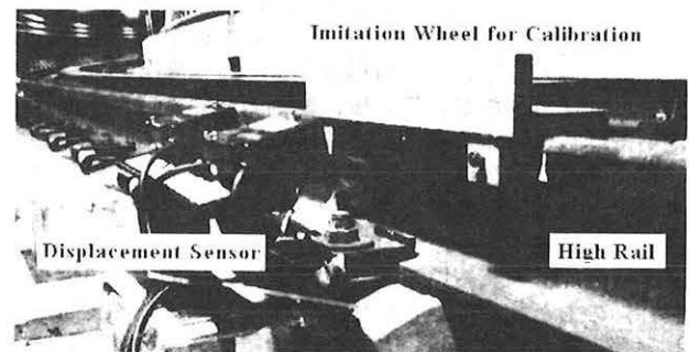
Fig.6 Wheel/Rail Displacement Sensor
