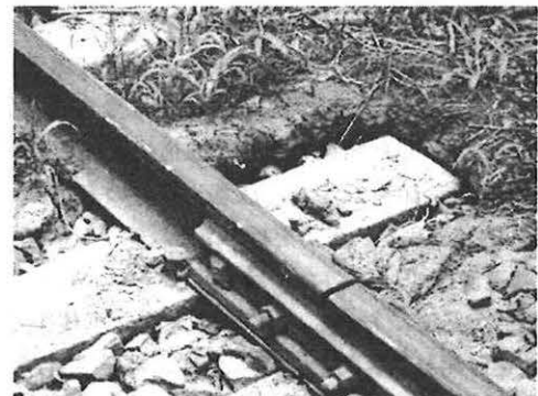
Fig.8 Loose Sleeper (2.3km)
