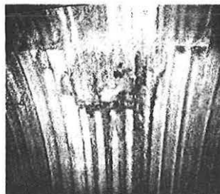
Fig.4 harmful alteration of steel deck
