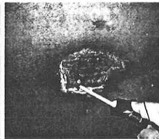
Fig.7 harmful alteration of GFRM
