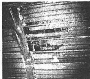
Fig.5 harmful alteration of liner plate
