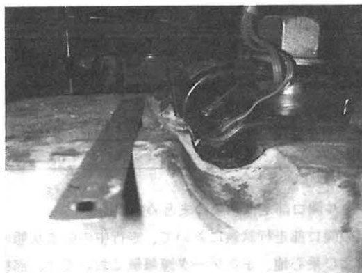
Figure-4 Destruction situation of PC sleeper receiving stopping
