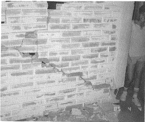
Photo5 Fracture of a Brick Wall with a Frame (Chile Earthquake 1985).
