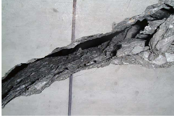
Photo 1 Crack surface of high-strength concrete
