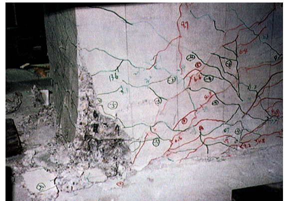
Photo 1 Specimen 1 Damage at Base
