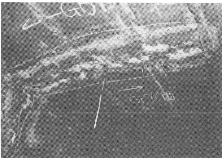
Fig. 5 Leaking water due to unfilled portion of grout
