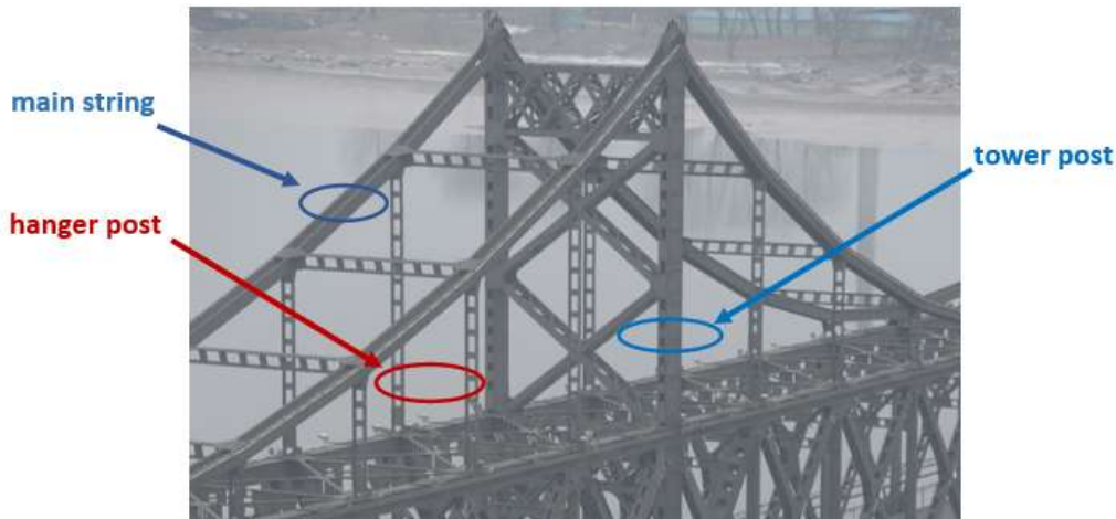
(a) Suspension strings of Yalu river bridge (Photo taken by Prof. Y. TAKAHASHI)
