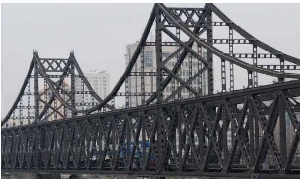
Fig.14 Truss members and suspension hanger strings of Yalu river bridge (Photo taken by Prof. Y. TAKAHASHI)
