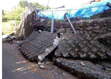
(e)練石積擁壁の倒壊 (西原村)
