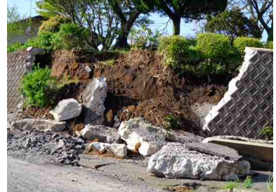
(f)練石積擁壁の倒壊 (南阿蘇村)
