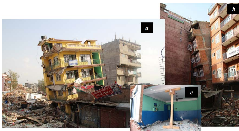
Fig.3.7 At Gongabu, RC frame buildings were tilted (a,b). A shear crack in the first flower (c)
