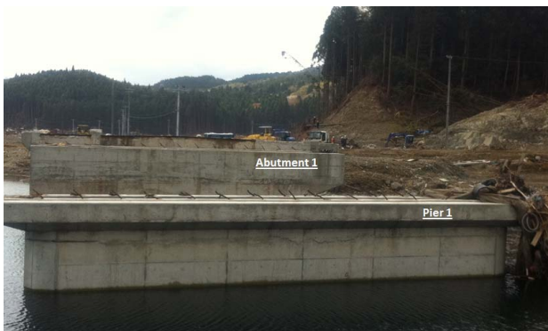
Figure 6 Bent dowel pins at pier 1 and abutment 1 (Date & location: May 4 th , 2011, 38.647156, 141.436973)
