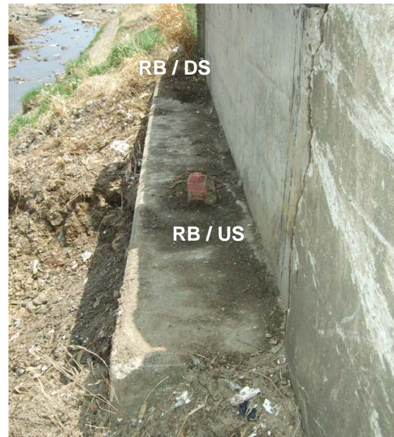
Figure 11 Line bearings on the right abutment: A rusty bolt for the RB/DS bearing was remaining on the lower flange of I-beam indicating that the friction between the anchor and the concrete had been loosened already.
