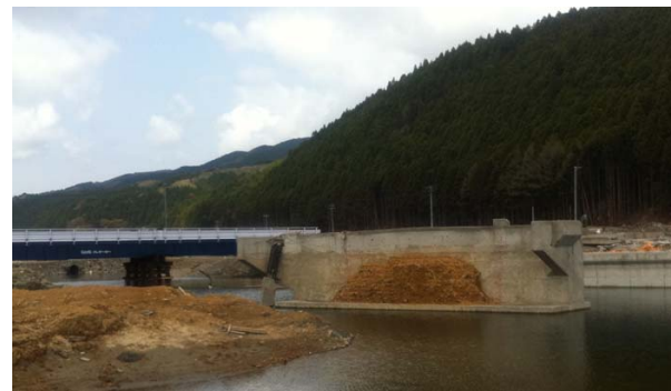
Figure 7 Eroded backfill at abutment 1 (Date & location: May 4 th , 2011, 38.646771, 141.437469)
