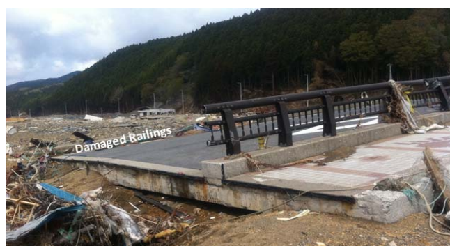
Figure 9 Damaged railing at west side of span 1 (Date & location: May 4 th , 2011, 38.646611, 141.439671)
