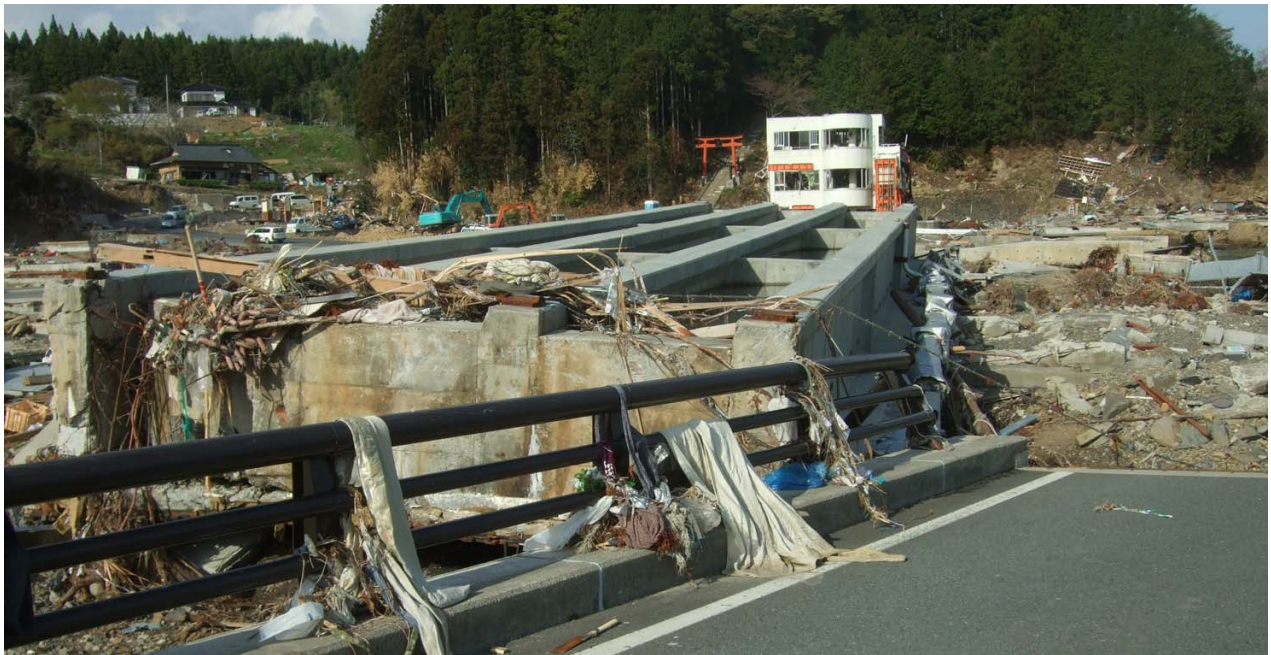
Figure 16 Bridge deck lying upside down showing lattice work of beams (Date & location: May 4 th , 2011, 38.716373, 141.522153)
