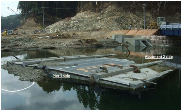
Figure 4 Displaced Deck 2 of Oritate Bridge (Date & location: May 4 th , 2011, 38.647134, 141.436868)
