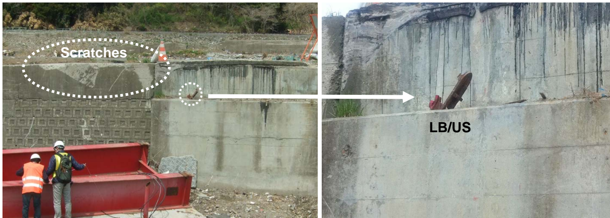
Figure 12 Broken line bearing on the upper stream side of the left abutment (LB/US) and scratches remaining on the left river wall (Date & location: May 4 th , 2011, 38.646726, 141.42659)
