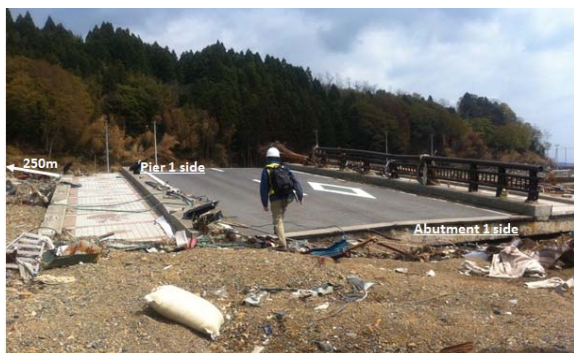
Figure 8 Displaced Deck 1 of Oritate Bridge (Date & location: May 4 th , 2011, 38.646589, 141.439437)
