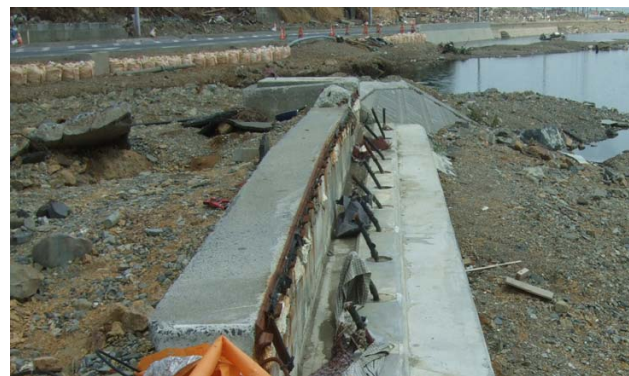
Figure 5 Bent dowel pins at abutment 2 (Date & location: May 4 th , 2011, 38.647134, 141.436868)
