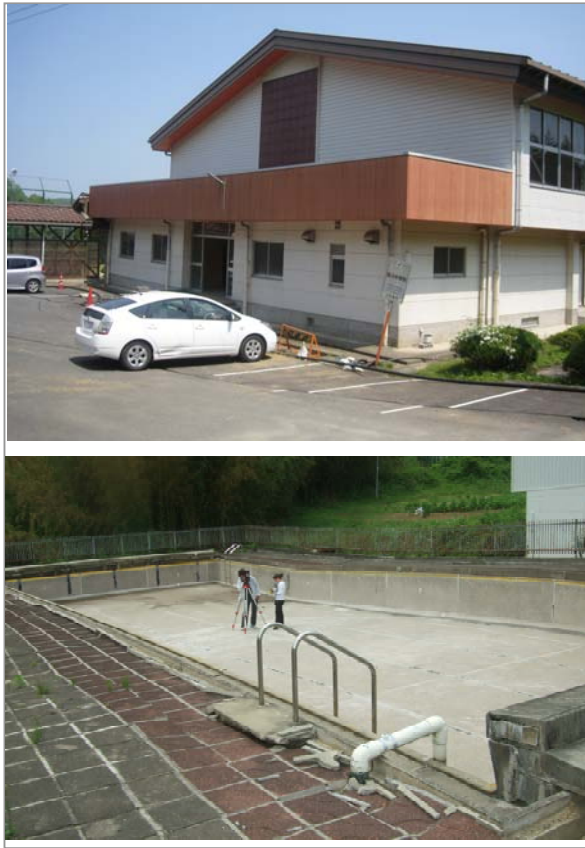
Figure 9. Idosawa Fault passing exactly under the gymnasium building (upper photo) and swimming pool (lower photo) of Tabito Junior High School, tilting and deforming the structures ( 36^{\circ}57'52.2'' , 140^{\circ}42'10.0'' )
