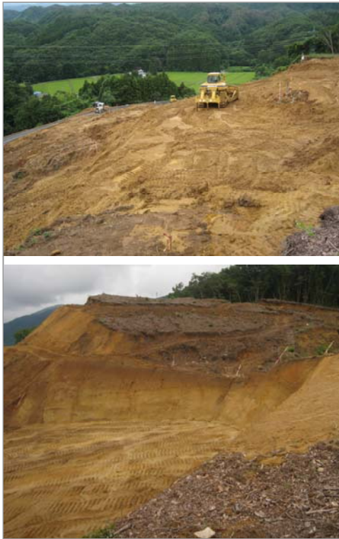
Figure 6. The landslide mass is re-profiled to an apparent stable configuration for the purpose of road construction. Huge tension cracks (lower photo) are present along the top, showing the deep seated slip planes.
