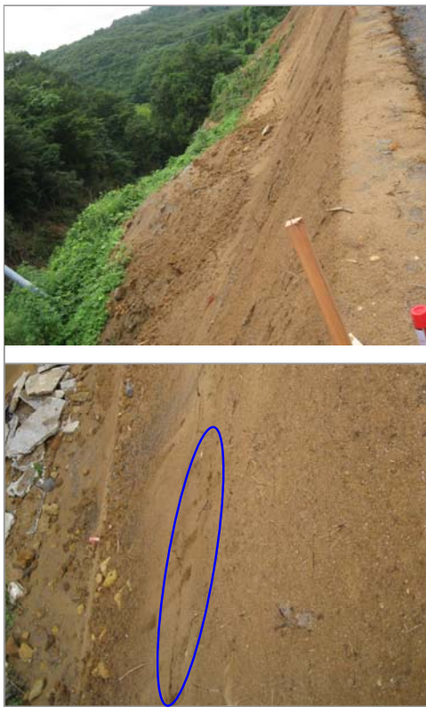
Figure 7. Embankment of the road constructed on the landslide mass (upper photo). Small scale cracks were observed near the base of embankment even during construction (lower photo).
