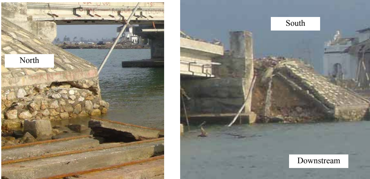
Figure 4. Scouring of approaches near abutments, downstream side
