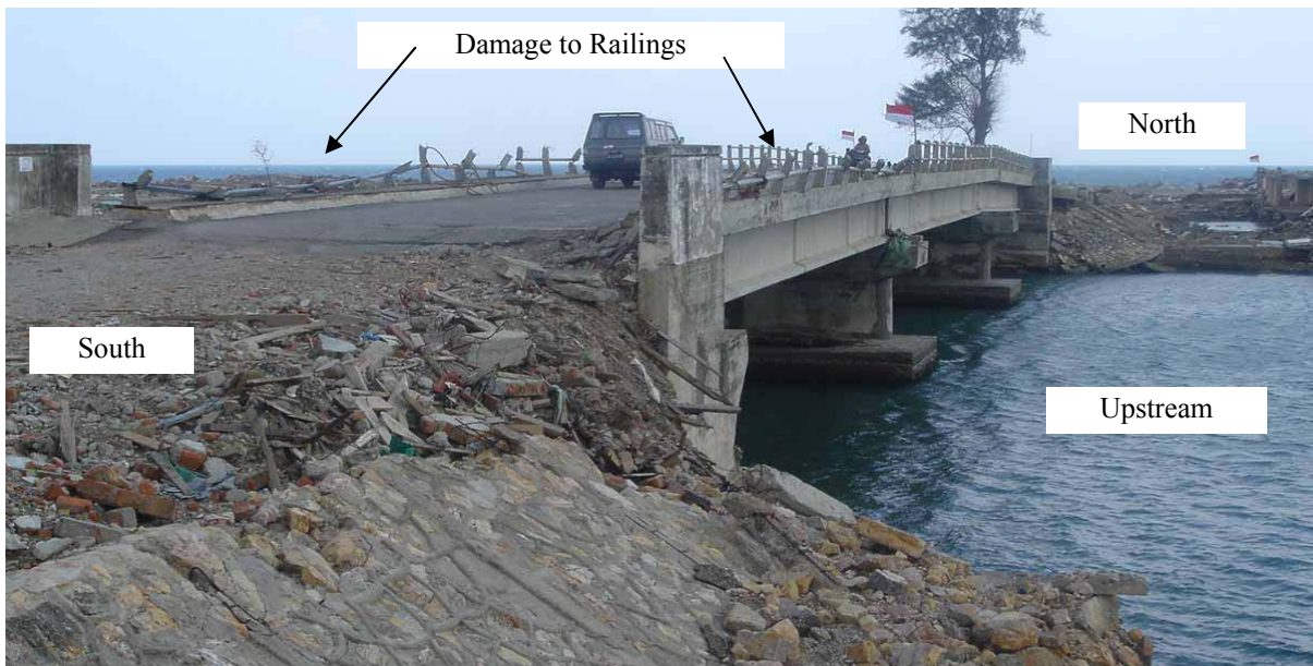
Figure 5. Damage to railings (also showing scourings at the upstream side)
