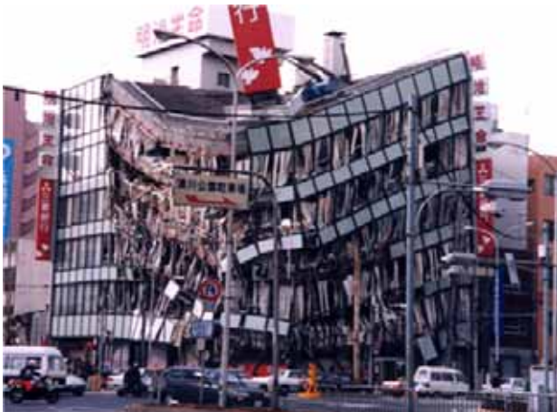
Figure 14 Ground-level soft-story collapsed building during Kobe Earthquake, 1995 (by K. Meguro)
