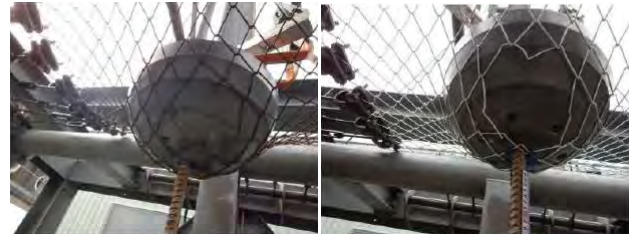
(a)劣化材 (b)新品材
