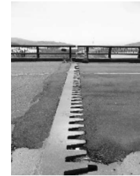
(c) A1橋台遊間の異常
