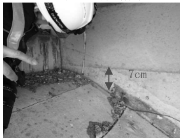
(e) A1橋台法面の沈下(7cm)
