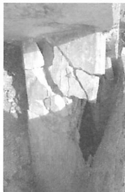
(e) Shear Failure of Pile Head
