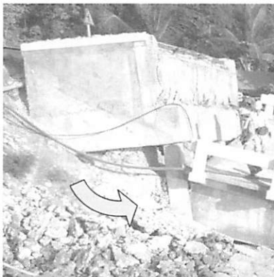
(d) Residual Inclination of Northeast Abutment
