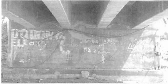
(a) Damage to Girder-Abutment Connection
