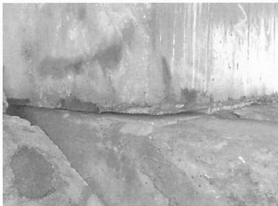
(c) Gap at Abutment-Footing Connection
