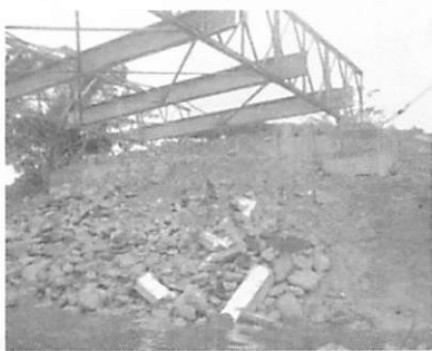
Superstructures had already been demolished and a temporary bridge was constructed when authors visited.
