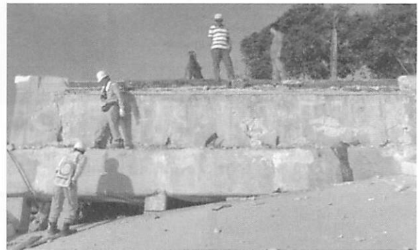
(f) Traces of Collision between Parapet and Girders
