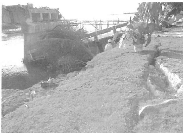
Photo 2 Big crack of embankment heading for northeast abutment
