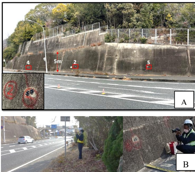
Figure 6: A. Retaining wall with an inset image of the target at position 2. B. Taking a photo from an arbitrary position
