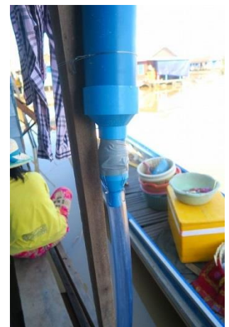
Fig.13 The joint portion of the gutter and the hose
