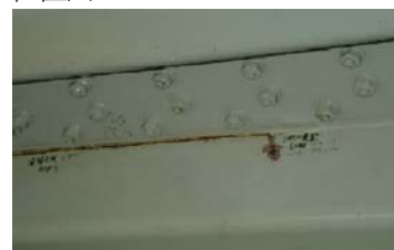
(c) き裂発生状況
