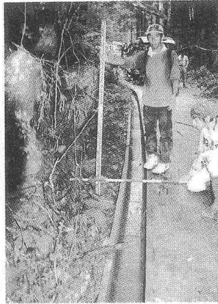
写真-5 側溝横の斜面の洗掘
