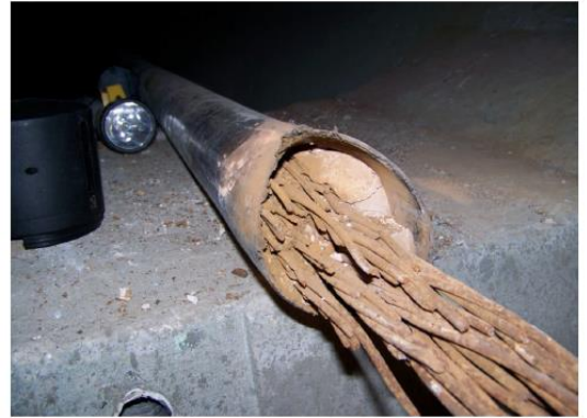
図-1 PC 鋼材の破断 (Varina-Enon 橋) 1)
