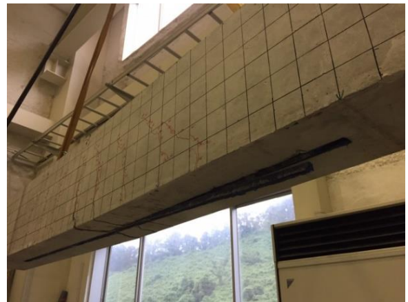
Fig. 3 Peeling status of reinforcing material SR48-1
