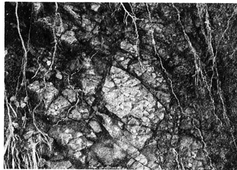
Photo 1. The complicated features of over-consolidated soil on a cut slope
