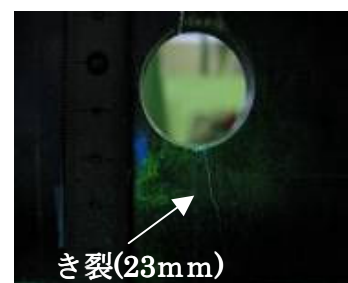
写真-1 SH-3 疲労き裂
