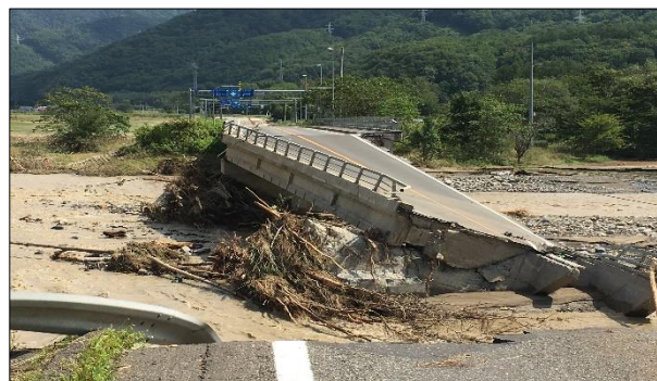
Figure 2. Riverbank Erosion induced bridge failure of a bridge along National Road 274, Nissyo Pass, Hokkaido, Japan. Photo Credit: Dr. Hiroaki Nishi, CERl (2016).
