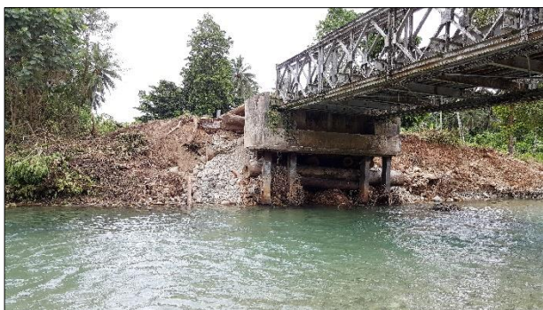
Figure 1. Riverbank Erosion induced bridge failure of Himutu Bridge, Boluminski Highway, New Ireland Province, Papua New Guinea. Photo Credit: Gibson Holemba (2016).
