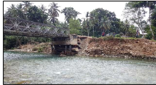
Figure 1 Flood-damaged Himutu Bridge, Boluminski Highway, New Ireland, Province, Papua New Guinea. Photo Credit: Gibson HOLEMBA (2016).
