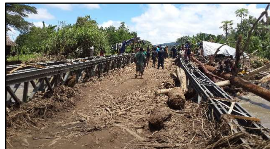
Figure 2 Flood-damaged Asas Bridge, Madang Province, Papua New Guinea. Photo Credit: Solomon Pela (2015)
