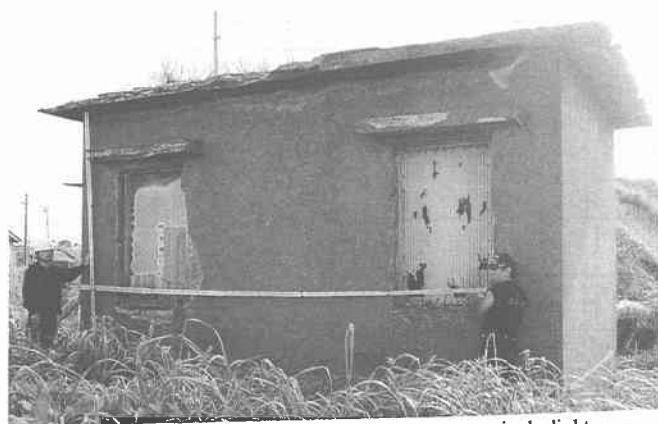
Photo-6 The east side which has deteriorated comparatively light
