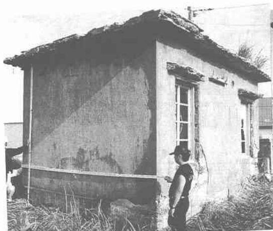
Photo-4 The north side which has deteriorated comparatively light
