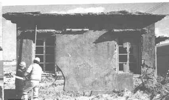
Photo-5 The west side which is deteriorated due to many cycles of freeze and thaw with sunshine in the afternoon in winter
