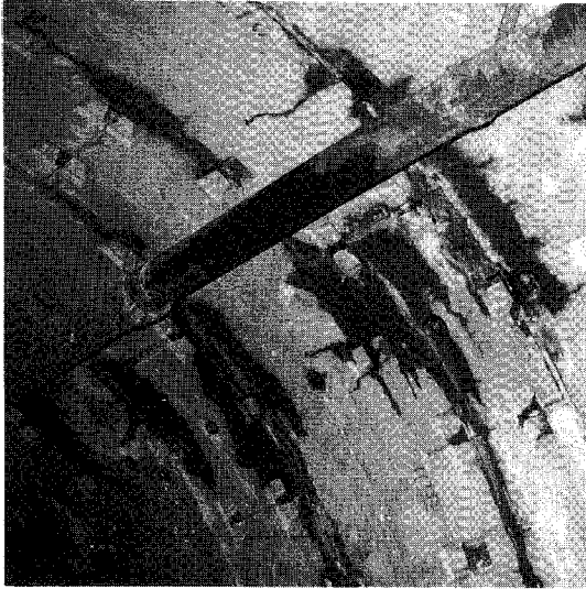
Photo.2 Cracks of segment linings on the ceiling
