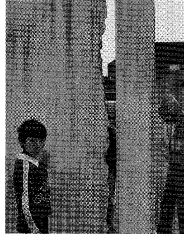
Photo 4 No Connecting Steel Bar between the Column and Wall (Equador Earthquake 1987).
