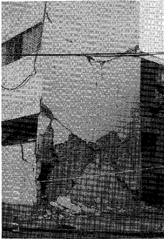
Photo 3 Typical Shear Cracks in a Brick Wall (Mexico Earthquake 1985).
