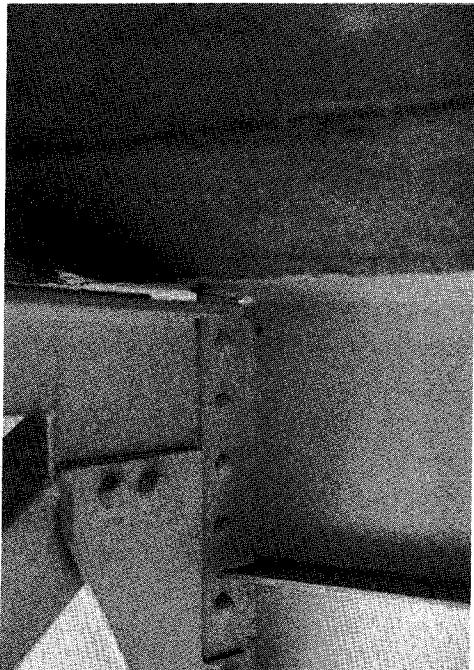
AB type+D type Crack
