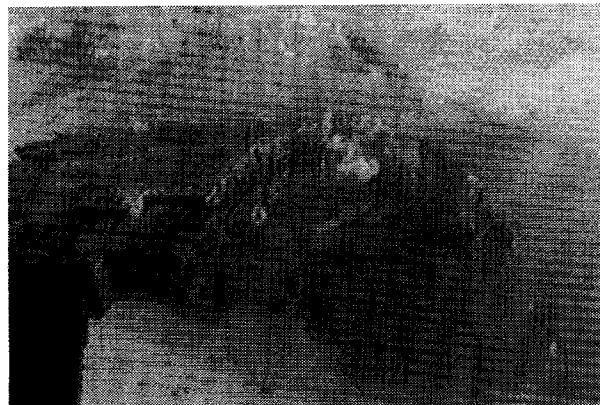
Photo 2 Collapse of arch stones (2).
