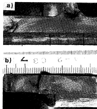
Photo 4 Fatigue fracture surfaces of tension flanges at the end of cover plates. Repair was made by groove weld.
