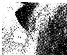
Fig. 19 Fatigue crack at the scallop of the vertical stiffener.
