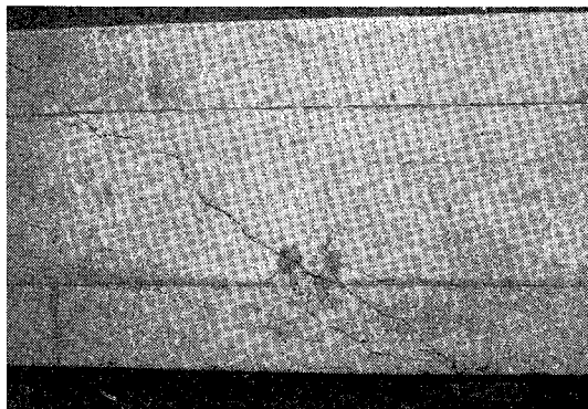
Fig. 14 Close-up view of failure in the second beam under the load of 120 tons at position C (the opposite surface of Fig. 4 (b)).
