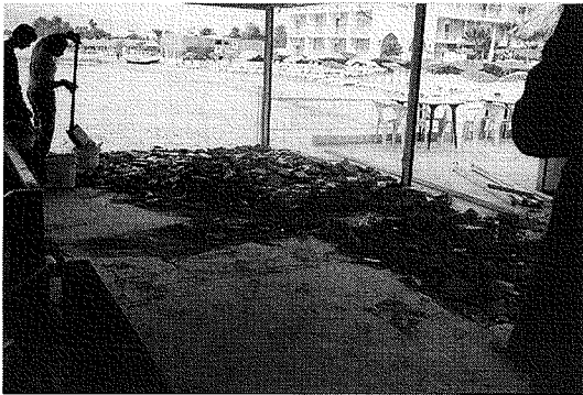
Fig.6 Ground deformation caused crushing of the floor slabs in structures built on the shoreline.
