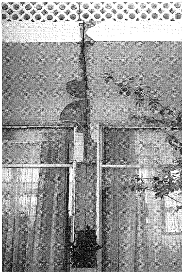
Fig.14 Narrow expansion vertical joints caused pounding between two wings for one of the hotels building.
