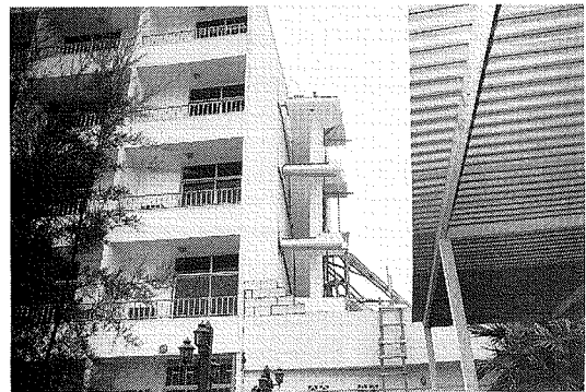
Fig.16 Separation of a poorly connected emergency exterior stair.
