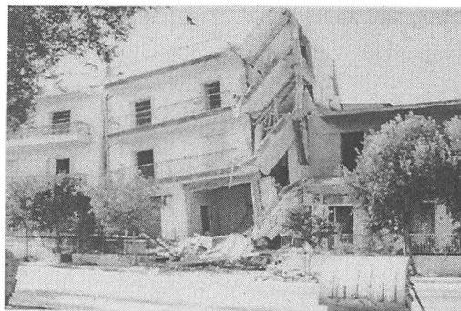
Photo 3 Damage due to pounding, Menidi.
