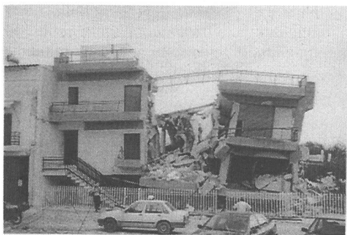
Photo 2 Column failure, due to the short-column effect, in a 5-story building in Ano Liosia.
