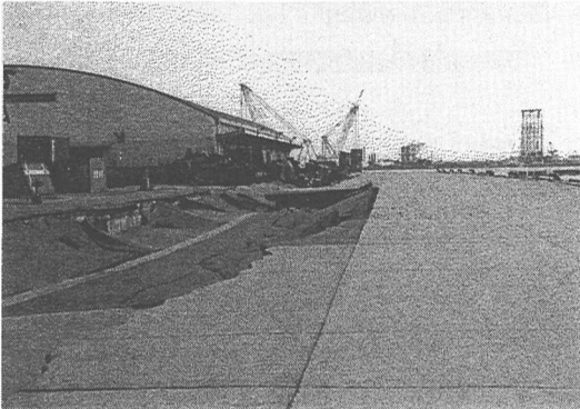
Photo 2 Deformation and settlement between caisson and cellular structures.
