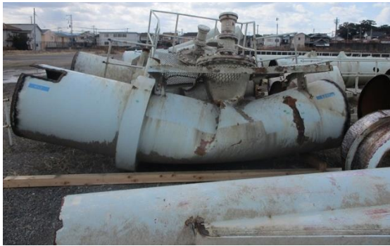
Fig.2 Wakayama aqueduct bridge failure
