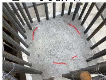
図-6 ひび割れ③
