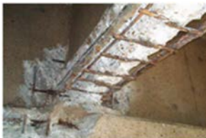
(c) 補強筋の腐食
