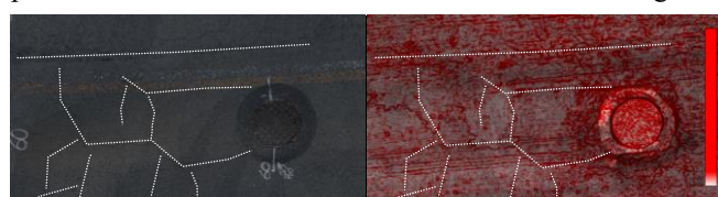
Fig. 6. Pavement cracks before (left) and after (right) milling 10cm of the pavement surface (white lines highlights the cracks visibility).
