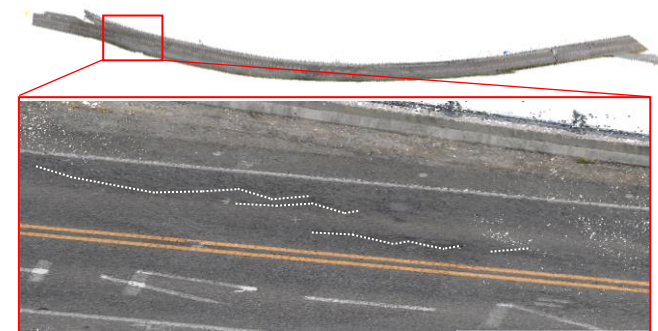
Fig. 5. Total area (top) and visible crack section (bottom) of Oura construction site 3D model by photogrammetry measurements.
