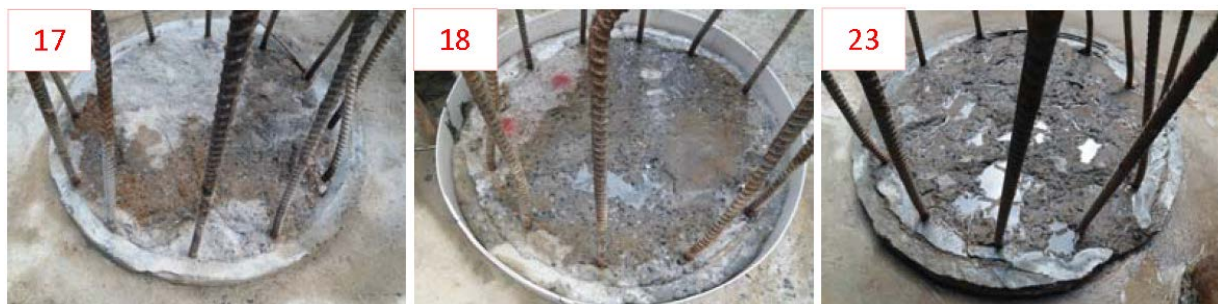
Fig. 3 Photo of water seepage at pile head
