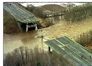
図-1 Schoharie Creek Bridge の落橋
