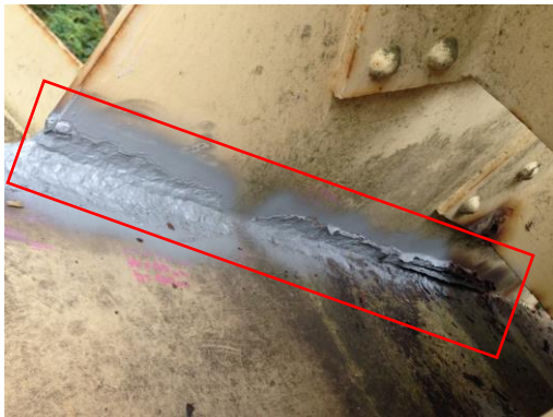
Fig. 1 Frequently corroded location on gusset plate connection.
