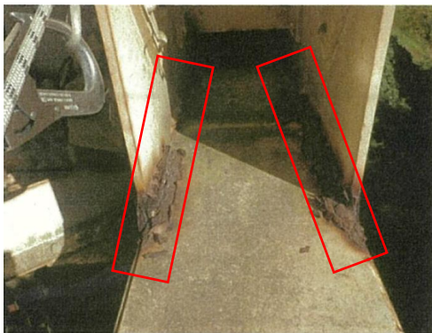
Fig. 1 Frequently corroded location on gusset plate connection.
