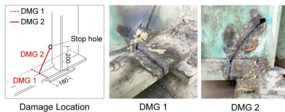
Fig. 3 Artificial damage of plate girder.
