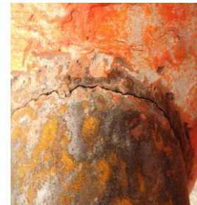
Fig.2 Example of crack
